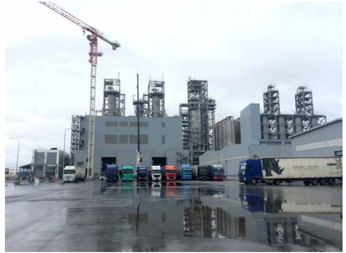
HDPE: Extrusion Structure. Lift commissioning to be started and punch clearance in progress
