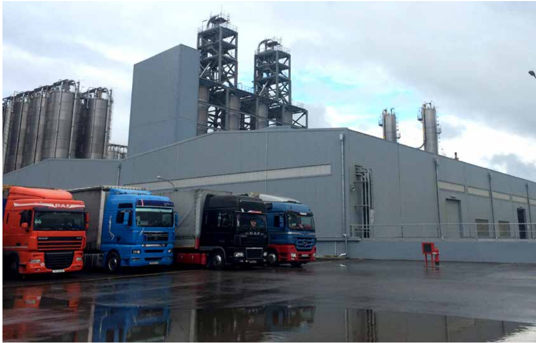
HDPE: Bagging & Packing. Punch clearance in progress
