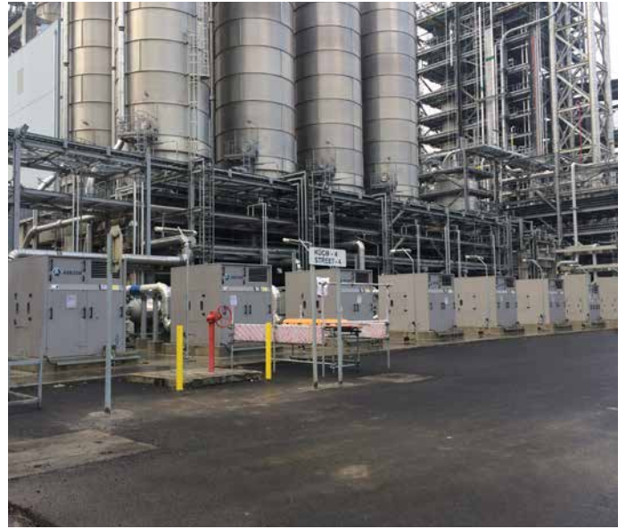
HDPE: Pellet blower package space for logistic conveying. Punch clearance in progress
