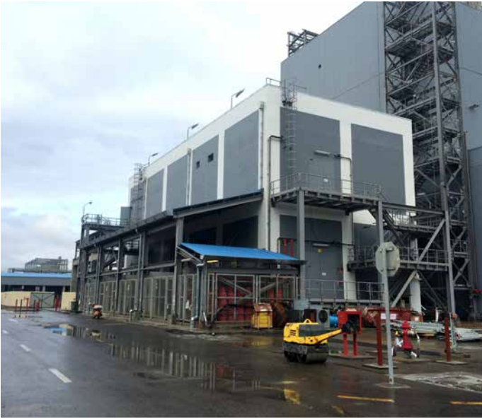
HDPE: Electrical Substation. HVAC Functional and performance test to start
